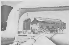
ONE OF the oldest buildings in the refinery, No. 2 Acid Contact Plant shows a partly stripped roof in the above photo. Workers are dismantling the building. It was built about January, 1936, and was shut down Dec. 22, 1960 after thirty three years in operation.
